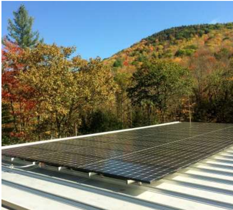
Photovoltaic installation at the Highway Garage
